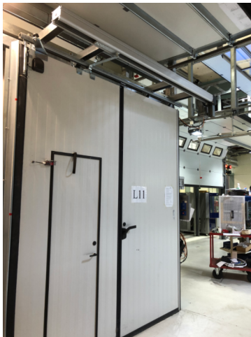
Figure 5.1: Original drive system.
