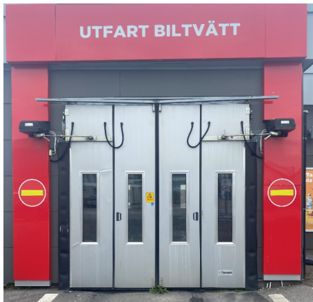
Figure 3.28: Side mounted motors on a car wash.
