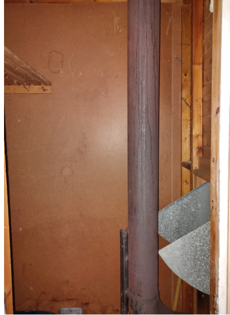
Flue heating the drying room.
