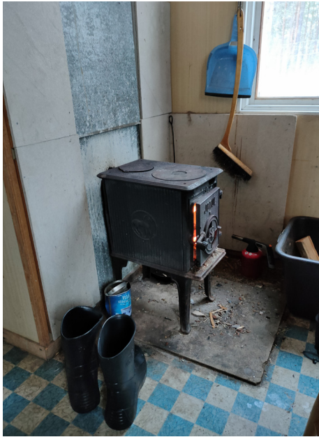
Jötul wood stove with a hob.
