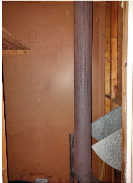
Flue heating the drying room.
