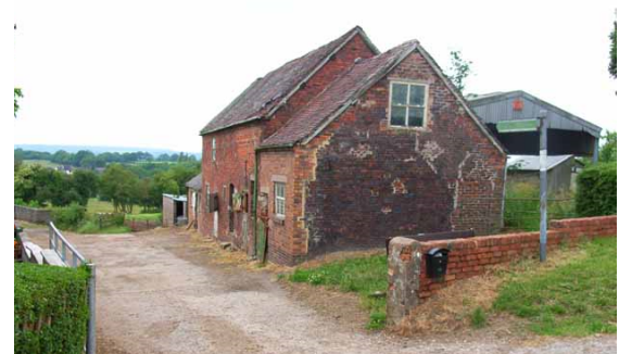
Building in the UK with poor building envelope (Unknown Author, licensed under CC BY-SA-NC)
