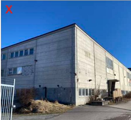
Figure 86. a building with bad conditions
