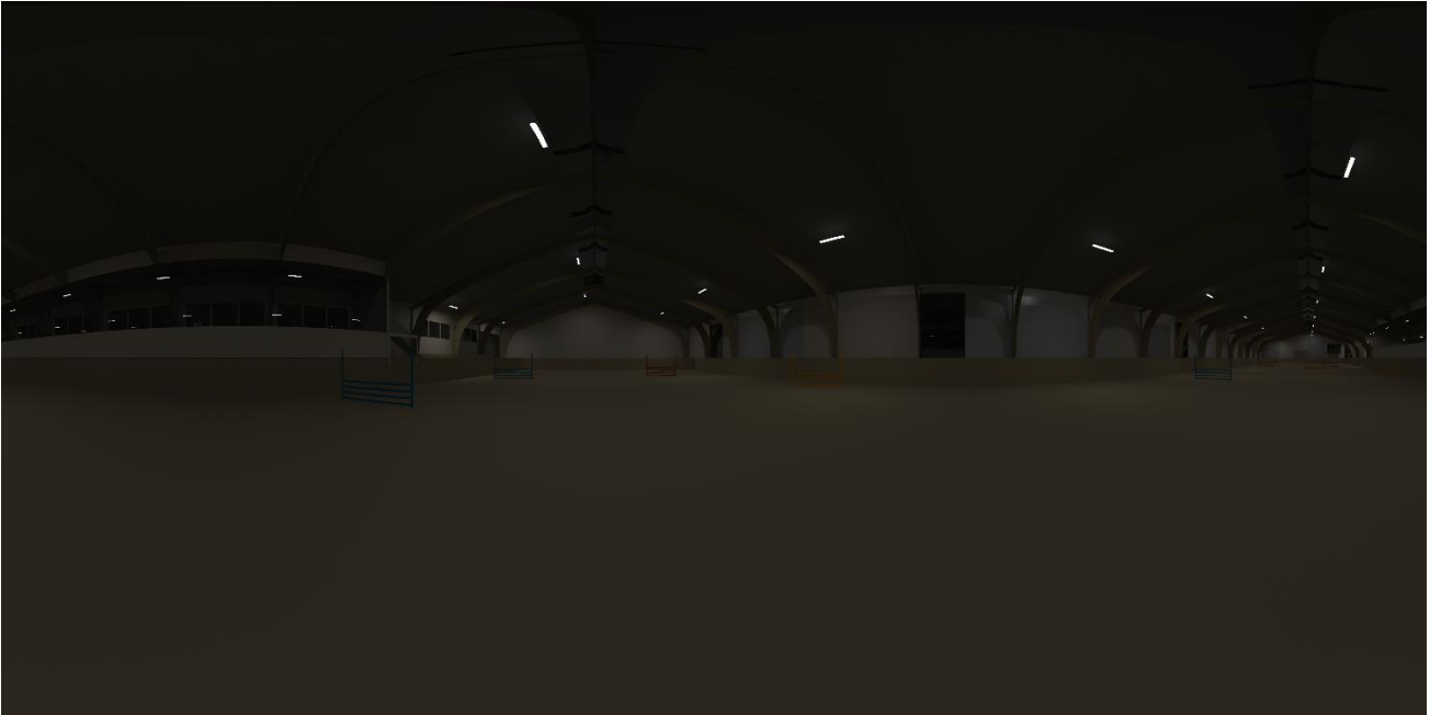
Figure 19: An equirectangular rendering with the proposed security lighting of the riding hall by installing fewer luminaires with higher power (30 lux environment).
