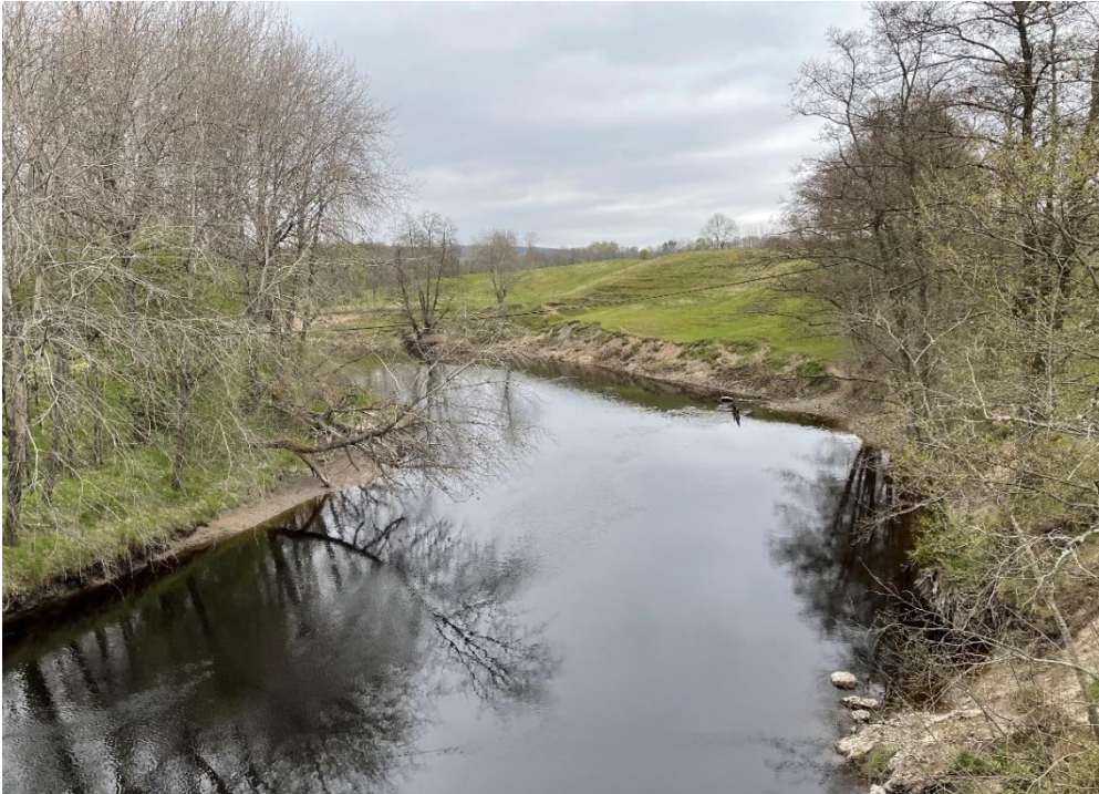
Figure 12. An example of typical erosion problems at Viskan causing trees to fall into river at upstream
