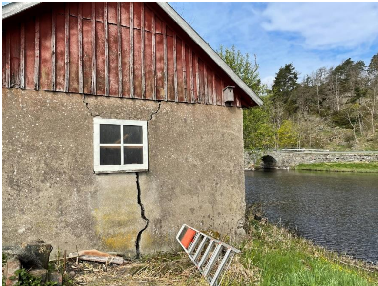
Figure 14. One of typical erosion problems at Viskan causing a house crack at downstream
