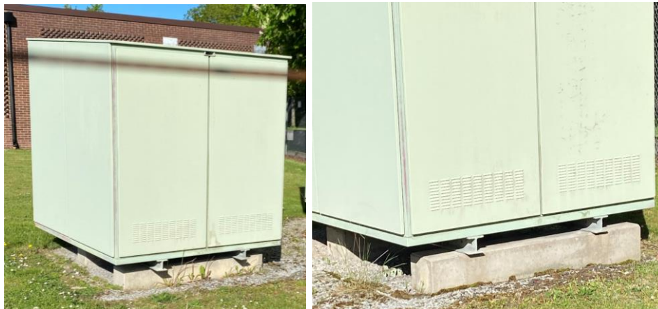
Figure 18: Industrial equipment supported by I-beams (Photo: Daniel Rundstöm).
