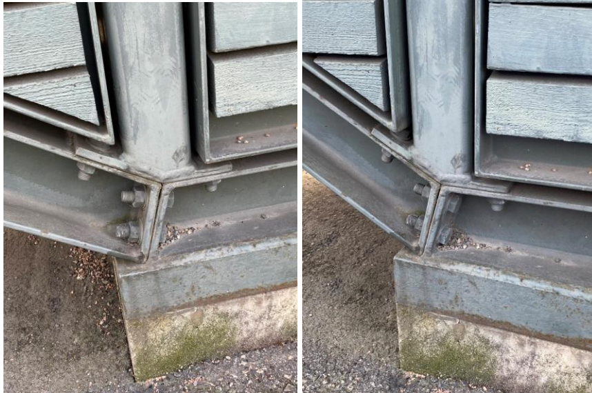
Figure 21: Two joined U-beams in a close to 45-degree angle (Photo: Daniel Rundström).
