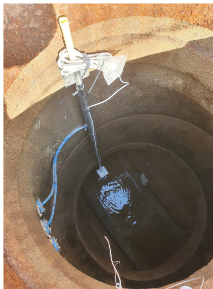
Figure 3.6: A picture of the installation of the sensor fluid flow measurement device at the 800 mm pipe TUAS_800 site of VA SYD. The installations are similar in all of the three pipes.
