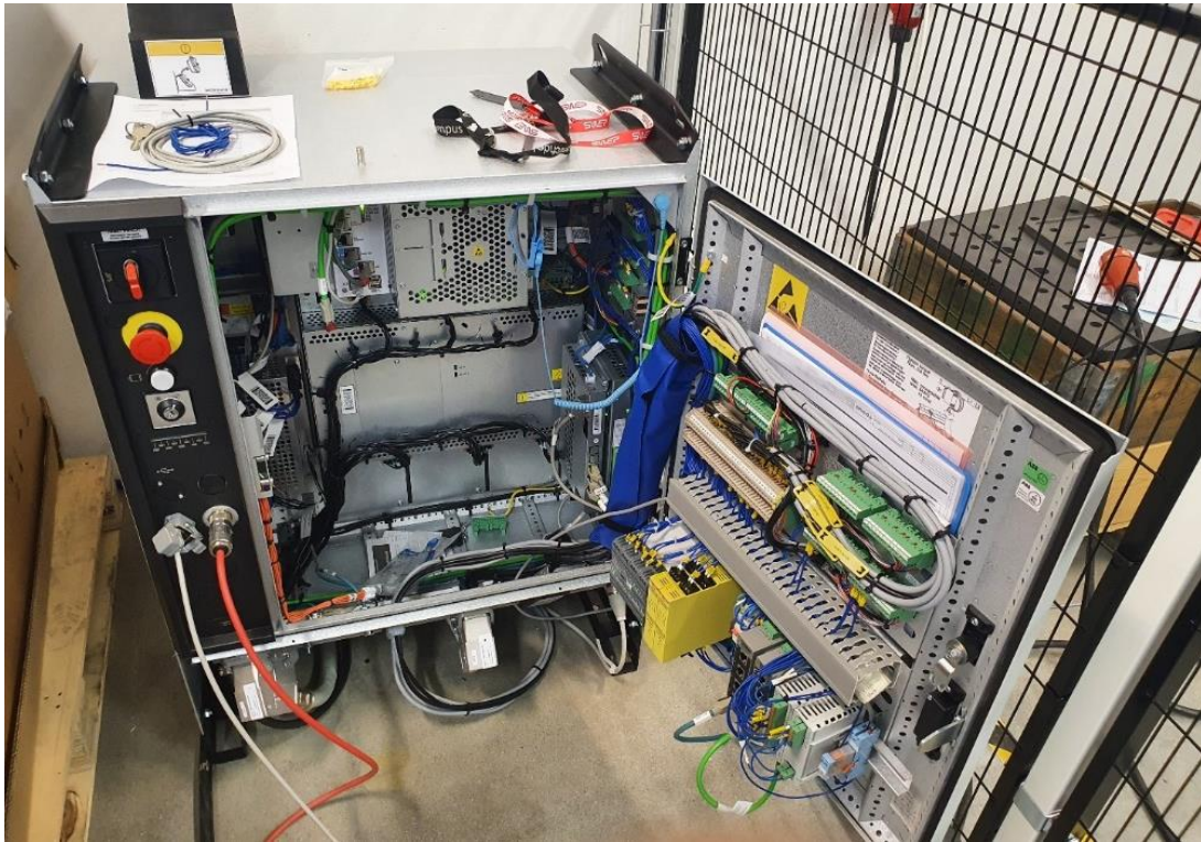
Figure 16: The IRC5 robot controller cabinet
