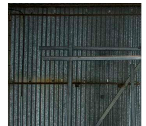
Facade plates from 1975, worn condition
