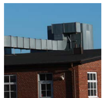
Mimicking the parasitical appearance of ventilation services.
