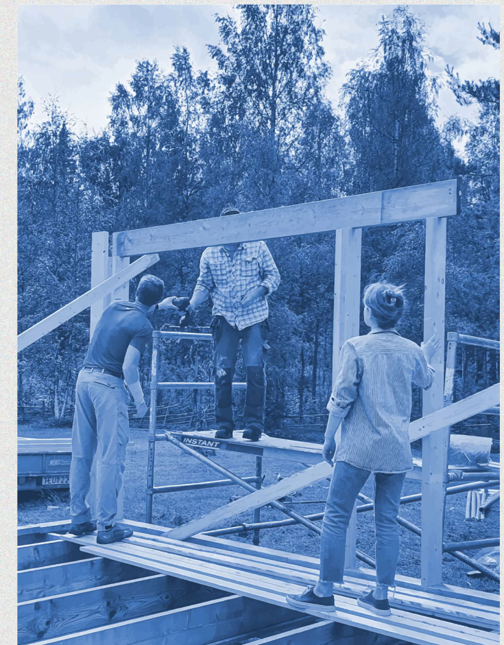
New foundation has been laid down with support from an old stone foundation found on site. Architect L, client J & his local woodworker brother P are working on the wood frame wall.
