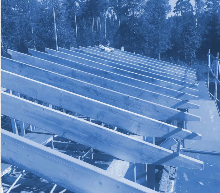
Ridge beam and rafters coming together. P is just finishing up some last screws.
