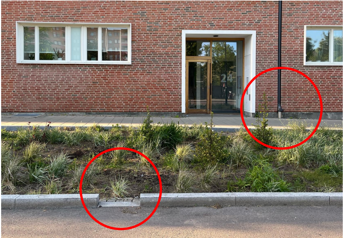
Picture 1 shows an inlet (on the left) without a sand-trap to keep sediment out of the raingarden, and an insufficient gradient hindering water catchment. Furthermore, the downpipe of the building (on the right) has not been connected to the raingarden. Picture taken by researchers.
