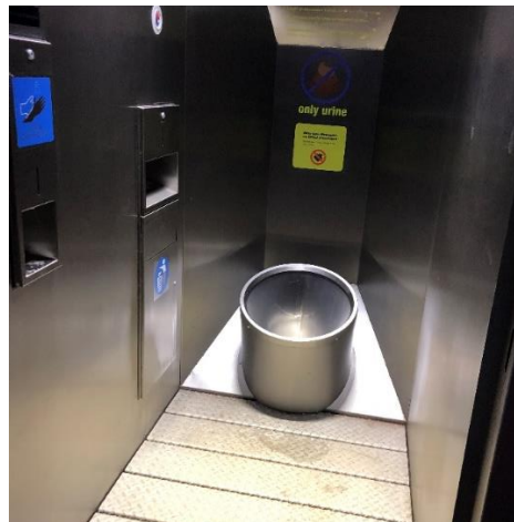
Figure 1-2 LooPi prototype developed and installed in Vienna
