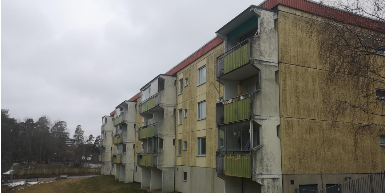
Picture 2 Worn out rental buildings in Tensta. (H. Koetsier, 2022)
