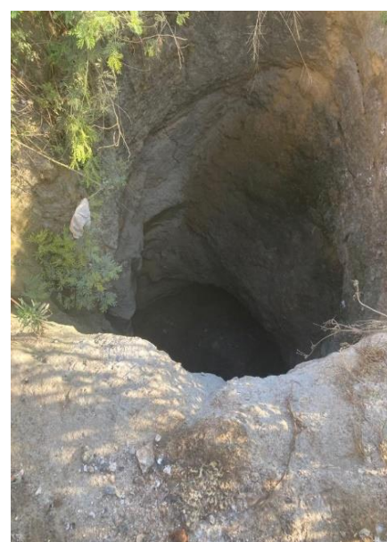
Figure 3: Sinkhole in Coronation.
