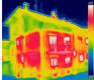
Figure 1 Building leaking energy
