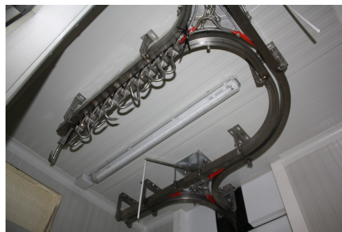
(b) tuna rail used in the chambers to move around large fishes in the room
