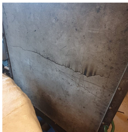
Figure 36: Crack in the back wall.
