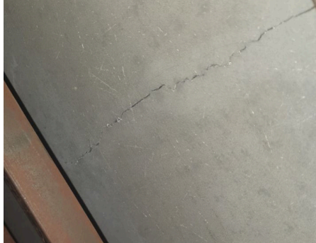
Figure 37: Crack below the room.
