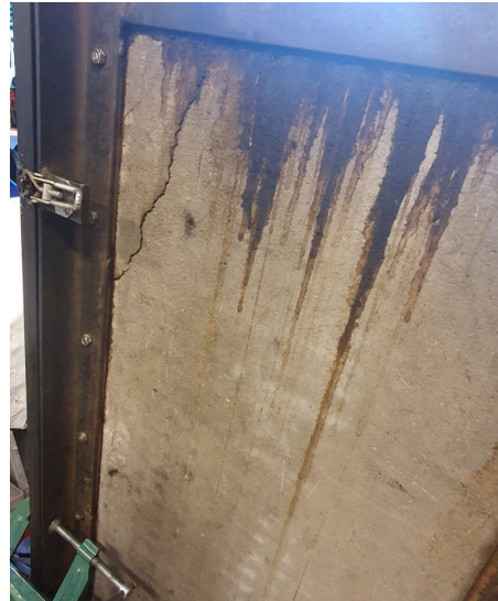
Figure 38: Crack in the corner where the burner was placed.
