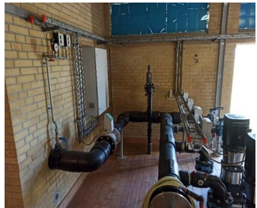
Figure 15. Waterworks at Lille Skensved.
