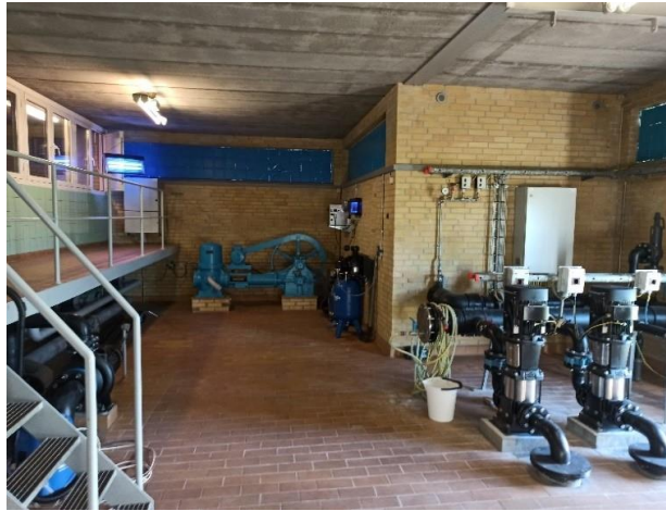
Figure 21. Waterworks at Lille Skensved
