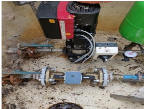
Figure 23. Booster station pump.
