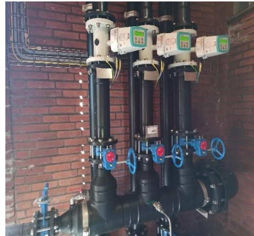
Figure 17. Main transmission pipes of Lille Skensved waterworks.
