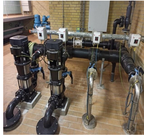
Figure 22. 4 parallel pumps at Lille Skensved waterworks.
