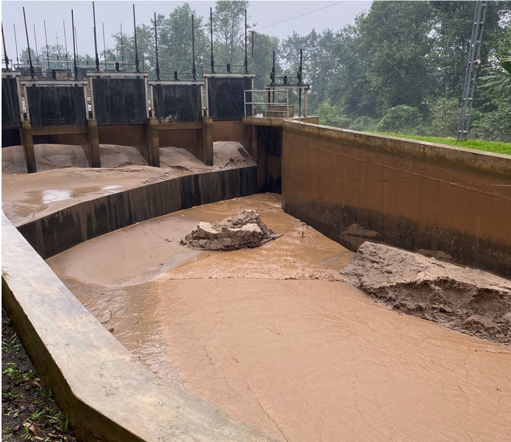
Figure 4-10 Sediment deposits in HPP channels.
