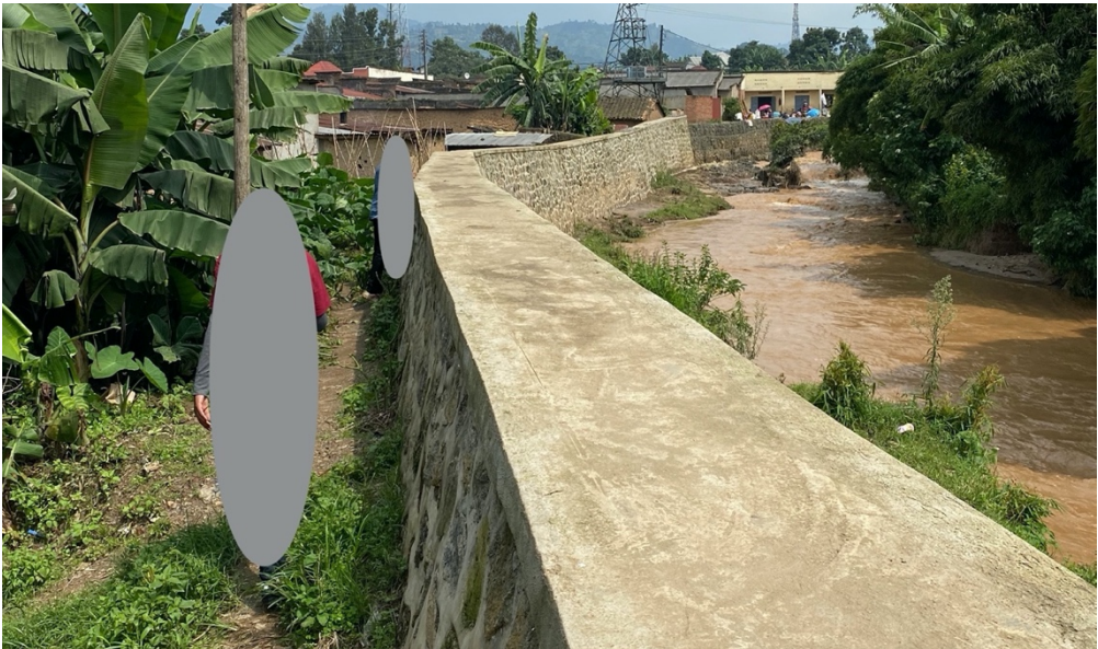
Figure 4-7 Retaining wall in Mahoko Village. In the photo grey ellipses are used for anonymisation.
