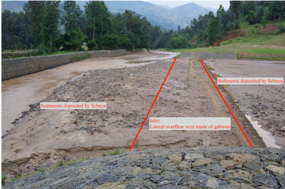
Figure 4-2 Sediment deposits at the inlet of the Sebeya lateral retention dike at Mahoko.
