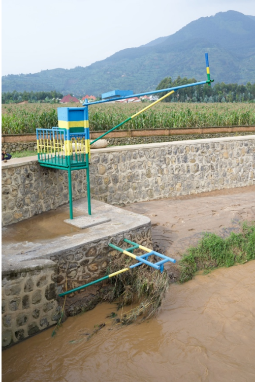
Figure 4-13 Nyundo telemetry station.
