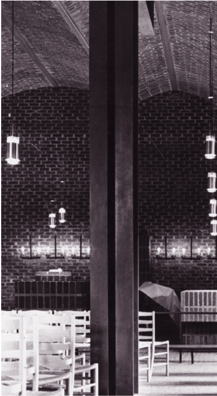
Figure 11: St Peters Church rusty steel Column, Klippan, Sweden 2018. (Source: Architectural Reveiw,2018:Online)
