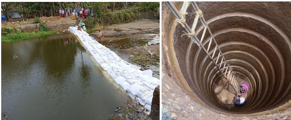
Figure 5: Water conservation works done under AUEGS in Wadakkanchery. Bund creation (left) and well construction (right) (Photos shared by the official in Wadakkanchery (left) and taken by the author (right), February 10, 2023)
