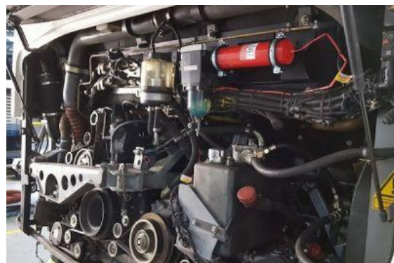
Figure 15 Aerosol system for LIB used in bus/coach engine compartment from RSL Fire [58].
