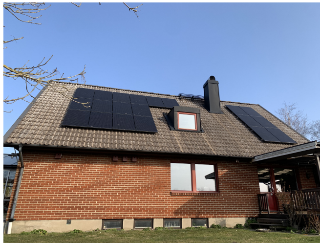
Figure 3.6: Residential PV system in Bara (photo: Annie Haraldsson, 2022)
