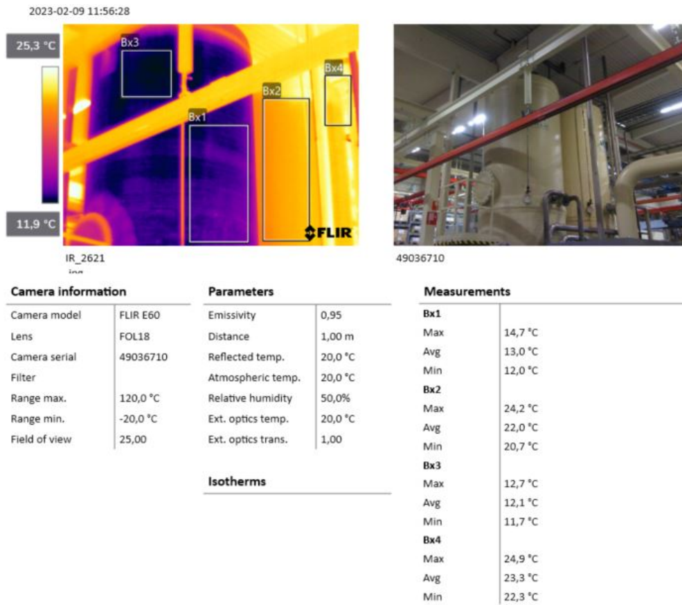
Figure 21 – IR picture of Cold (left) and hot (right) cooling tanks
