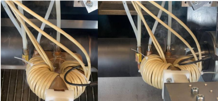
Figure 69 Failure of the coil
