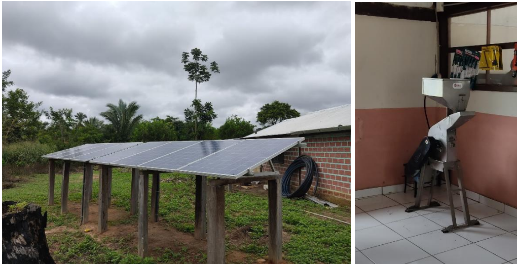
Figure 6-3. Facilities of the cusi producers. Left: solar panels installed for electricity. Right: cusi grinder Source: taken by the author
