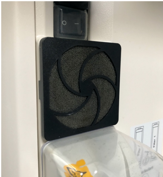
Fig. C4. Image showing the fan that needs to be cleaned from dust.
