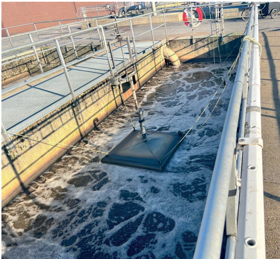
Figure 3.2.1. Arrangement of floating hood in the activated sludge unit for measuring N 2 O emissions at the Klagshamn wastewater treatment plant (Picture taken by me during the plant visit to Klagshamn WWTP).
