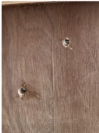
Figure 6. The picture shows the wall of the dryer chamber with drilled holes.
