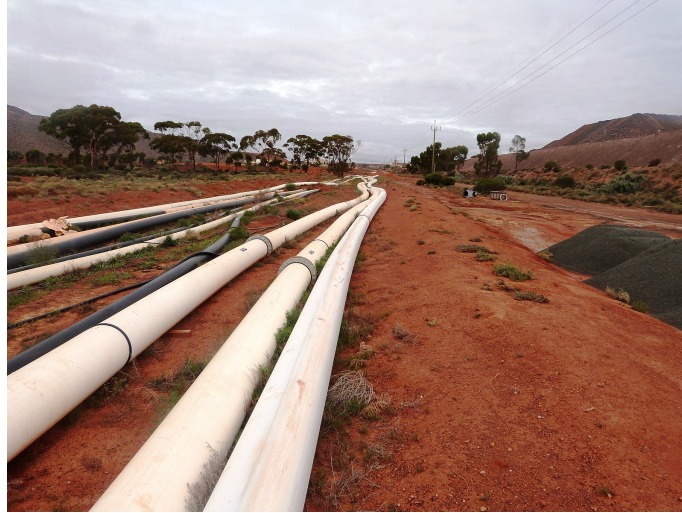
Figure 3 HDPE Pipeline used for water transportation
