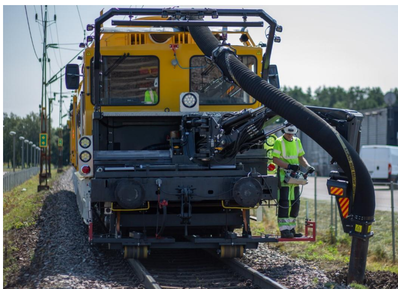
Figur 3, Vakuumsug modell "Railvac" (Foto: Johan Forslund, Railcare)
