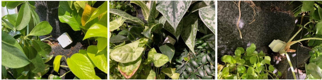
Fig.7: Detail of humidity sensors located in the green wall. Photography by Sahit TM
