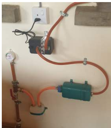
(b) The gas first flows through the (white) water removal box, second; through the (green) hydrogen sulphide removal box and lastly; through the (black) booster pump. A pressure gauge can also be seen to the left.
