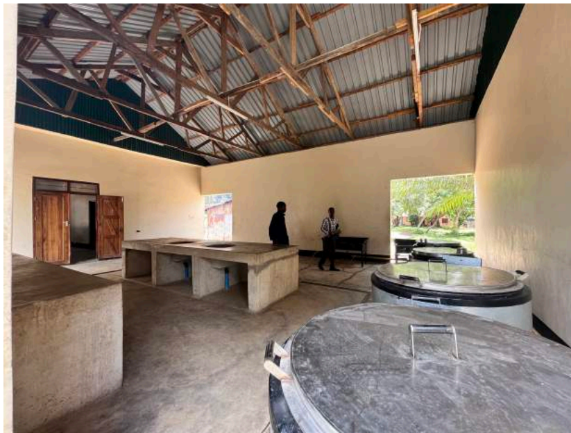
(d) The kitchen with gas ovens and stoves.
