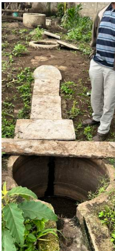
(a) Biogas plant system at Site 3.
