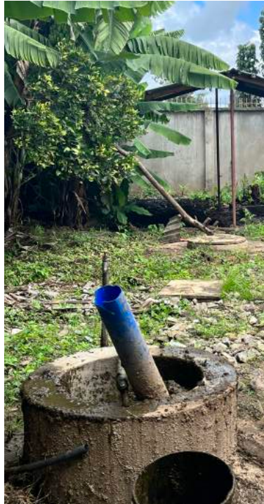
Figure 16: Biogas plant system at Site 2 (Lovisa Magnusson Ericsson, 2023).
