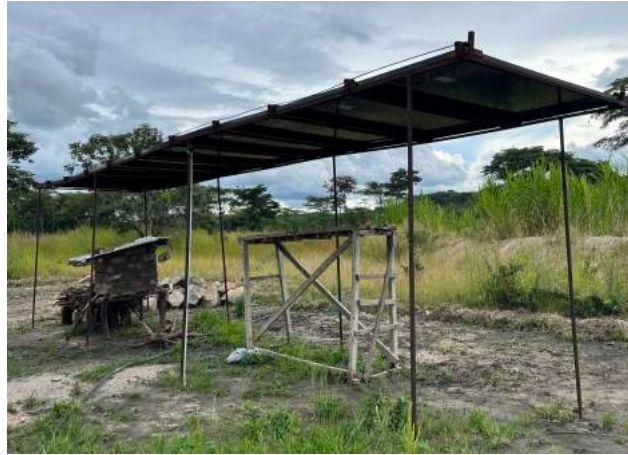
Figure 8: Solar PV installation at the Centre Director’s farming area (Lovisa Magnusson Ericsson, 2023).
