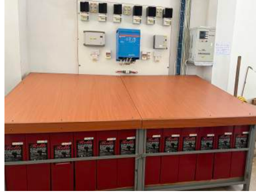
(b) The battery room at St. Ann Catholic Mission Hospital.
