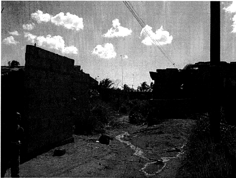
Picture 10.6 The roads are bumpy and narrow and the rainwater runoff is bad
