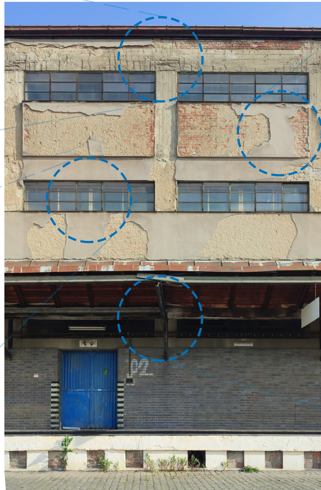
Image 33: Facade to the North, highlighting damages.
