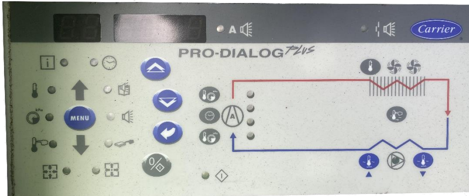
Figure 24 - The interface of the external cooling control panel.
