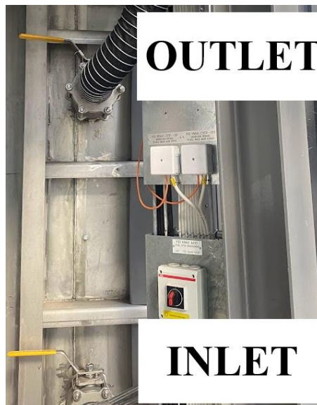
Figure 25 - The inlet and outlet of the flue gases found in zone 2.
