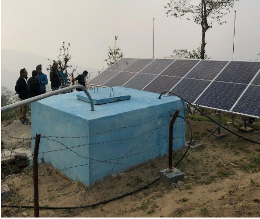
Figure 4 SWP: panels and tank. Photo taken by author.
