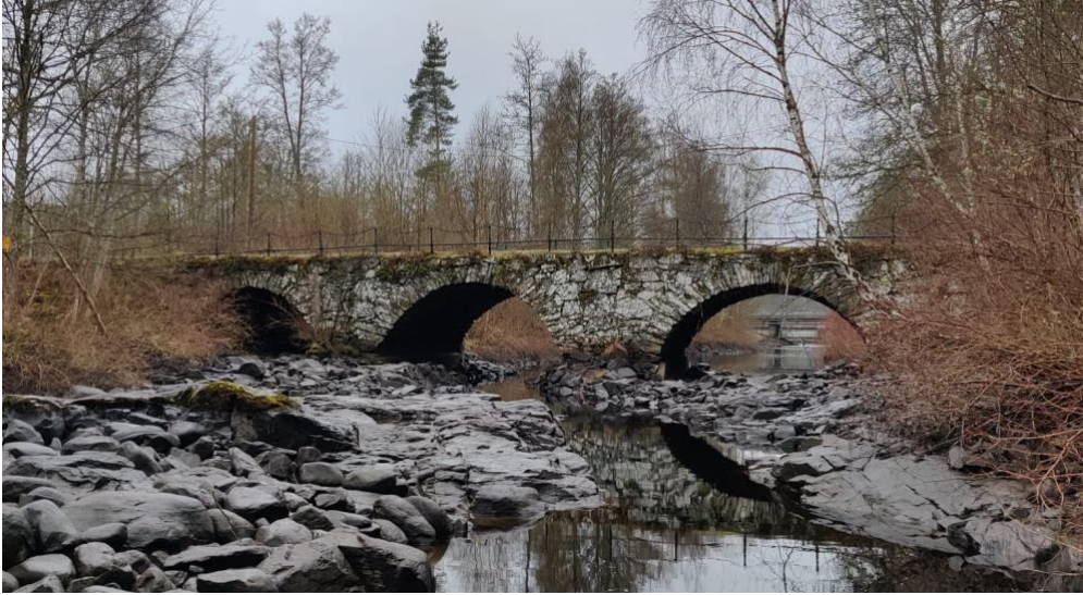
Figure 9. Photo of Hönjebro bridge, facing upstream. Highway 23 and a sluice gate of the Genastorp dam are visible through the rightmost arch.
