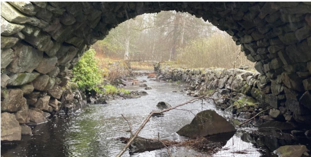
Figure 14. Upstream-facing view of Göta bruk channel, seen through the westernmost arch of Knut's Bridge.
