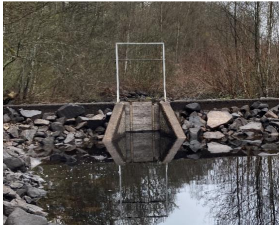
Figure 6. Downstream-facing (eastward) view of the northern sluice gate at Hönjarum dam during dry conditions.
