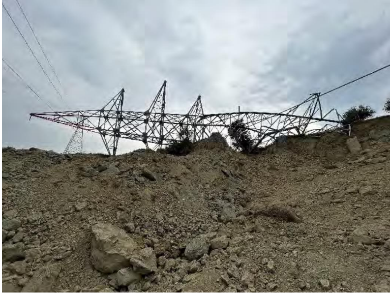
Figure 29. Collapsed steel transmission tower. Image from EERI and GEER (2023)
