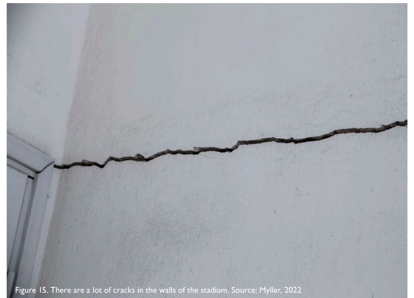
Figure 14. Cracks on the side of the stadium extension. Source: Mölsä, 2022
