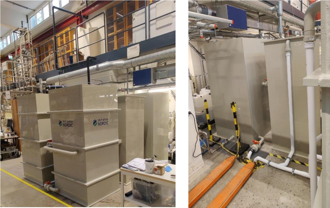
Figure 4.2. Overview of the pilot-scale rainwater treatment facility installed at Kemicentrum in Lund.
