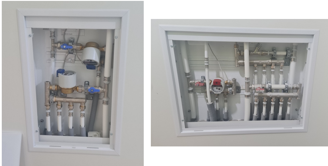
Figure 4.3. Individual Water Meters (Left: Cold and Greywater; Right: Hot)
