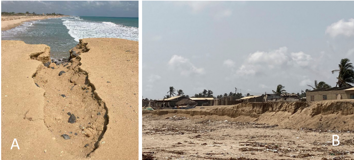
Figure 4A: Eroding sea-defence structure; B-Erosion at Otrokpe despite sea-defence structure (Photos taken by the author, 27 February 2024)
