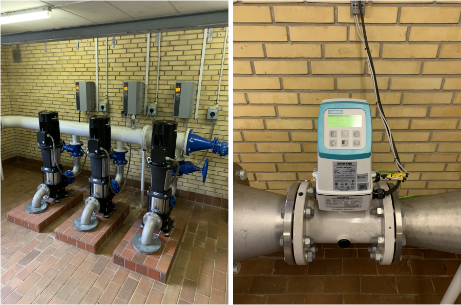
Figure 4.5. Pumps and flow meter in pump station Zone 1
