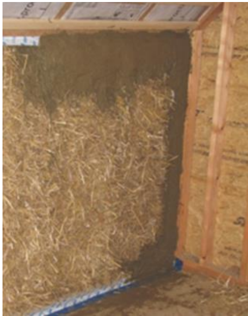
Figure 17: Connection of clay plaster to reinforced craft paper to prevent infiltration in the joist in traditional straw bale construction (ASBN, 2021)
