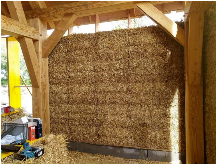
Figure 44: Post and Beam CUT wall on the exterior side of the post and beam construction in Kessel, Netherlands, lifted on concrete block foundation (A. Balatsoukas-Stimmin, personal communication, 17 January 2023)
