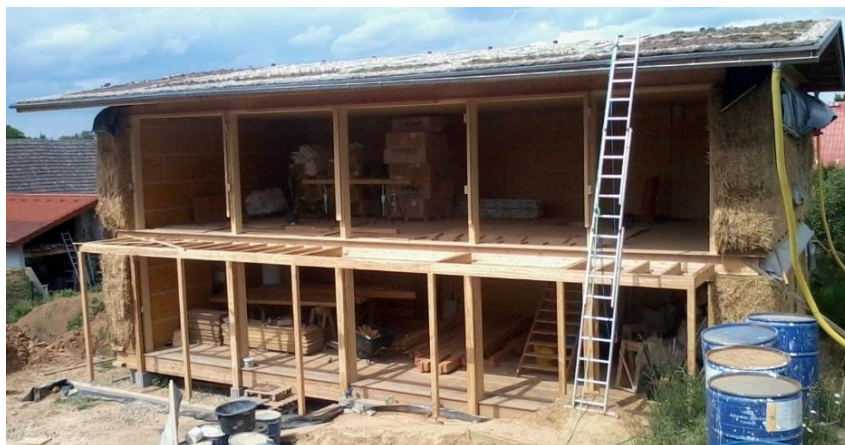
Figure 16: Load-bearing construction with OSB boards towards the interior to ensure higher levels of air tightness (CPD, 2017)
