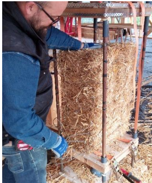
Figure 32: Small bale press using the tie down straps ready to use on building site (Respondent, personal communication, 23 March 2024)
