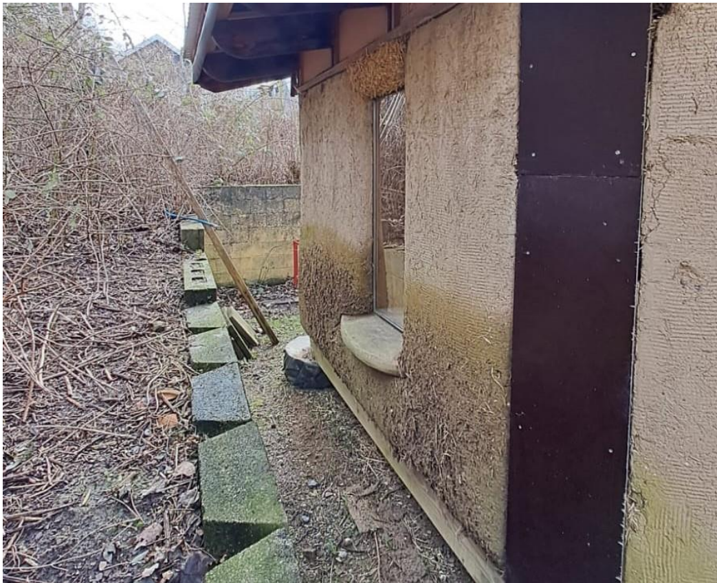
Figure 19: Moisture damage on two year old CUT Flexagone straw bale wall located in Denmark
