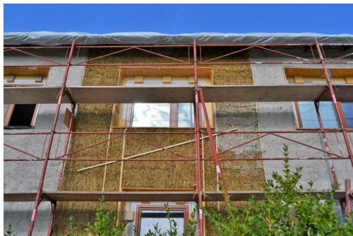
Figure 46: CUT wrapping of existing building using two possible methods in one wall (Gruber, 2020c)
