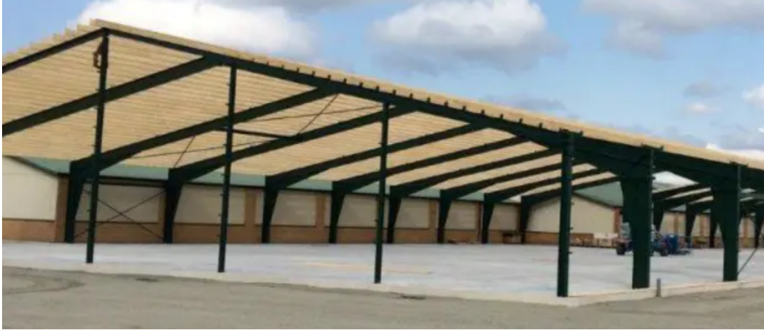
Figure 1.1: Construction of steel frames used in a hall building. Taken from https://www.lr-system.se/stalhallar/ .
