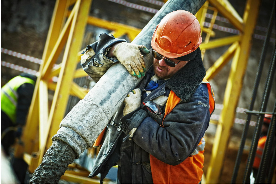
Figure 1.1: Manual control of the concrete pouring hose on a typical construction site, image by Yuri Kim [1].
