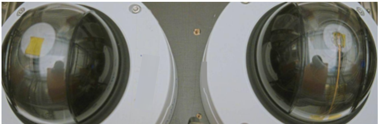
Figure 27: Image from test 1. Condensation can be seen in both cameras as light circles in the center of each dome.
